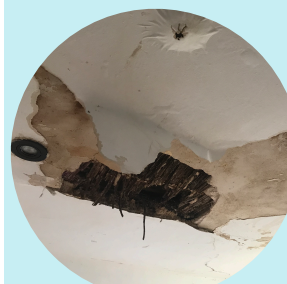
The hole in our ceiling
